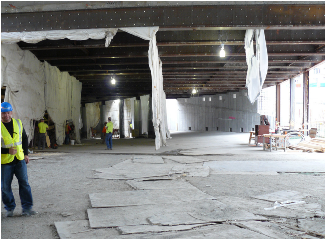
Figure 34: View on the Vehicle Security Center; entrance for vehicles on the right (own photography by Fraunhofer EMI)
